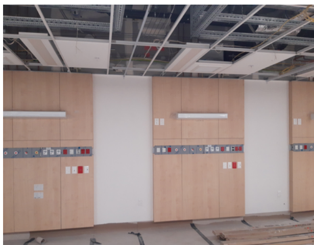
Medical service panels which will provide utilities to the patient beds.
